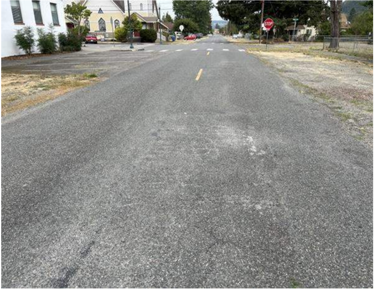
Figure 9. Alligator Cracking on Varner Avenue
