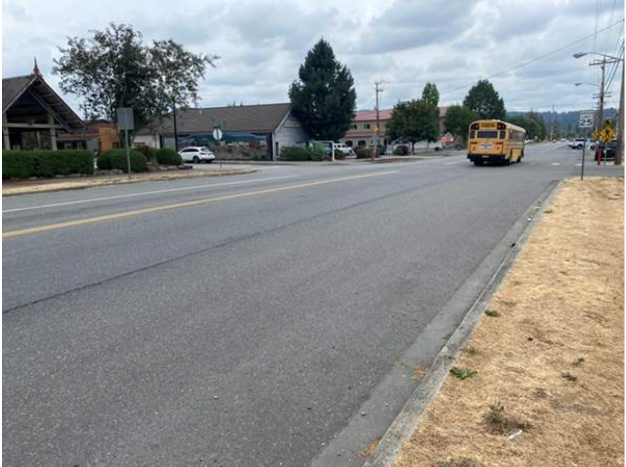
Figure 12. Longitudinal Wheelpath Crack along Calistoga Street
