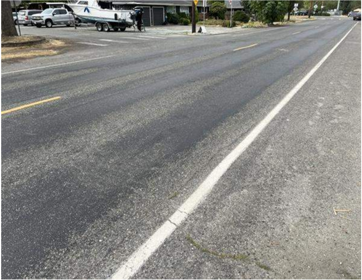
Figure 6. Rutting on Kansas Street
