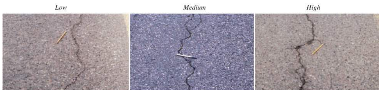
Figure 11. Longitudinal Wheelpath Cracking Severities
