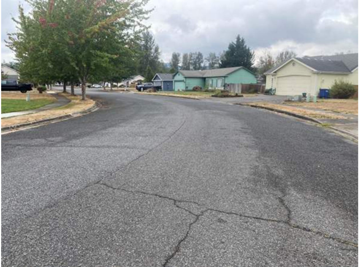
Figure 18. Transverse Cracks on Belfair Avenue
