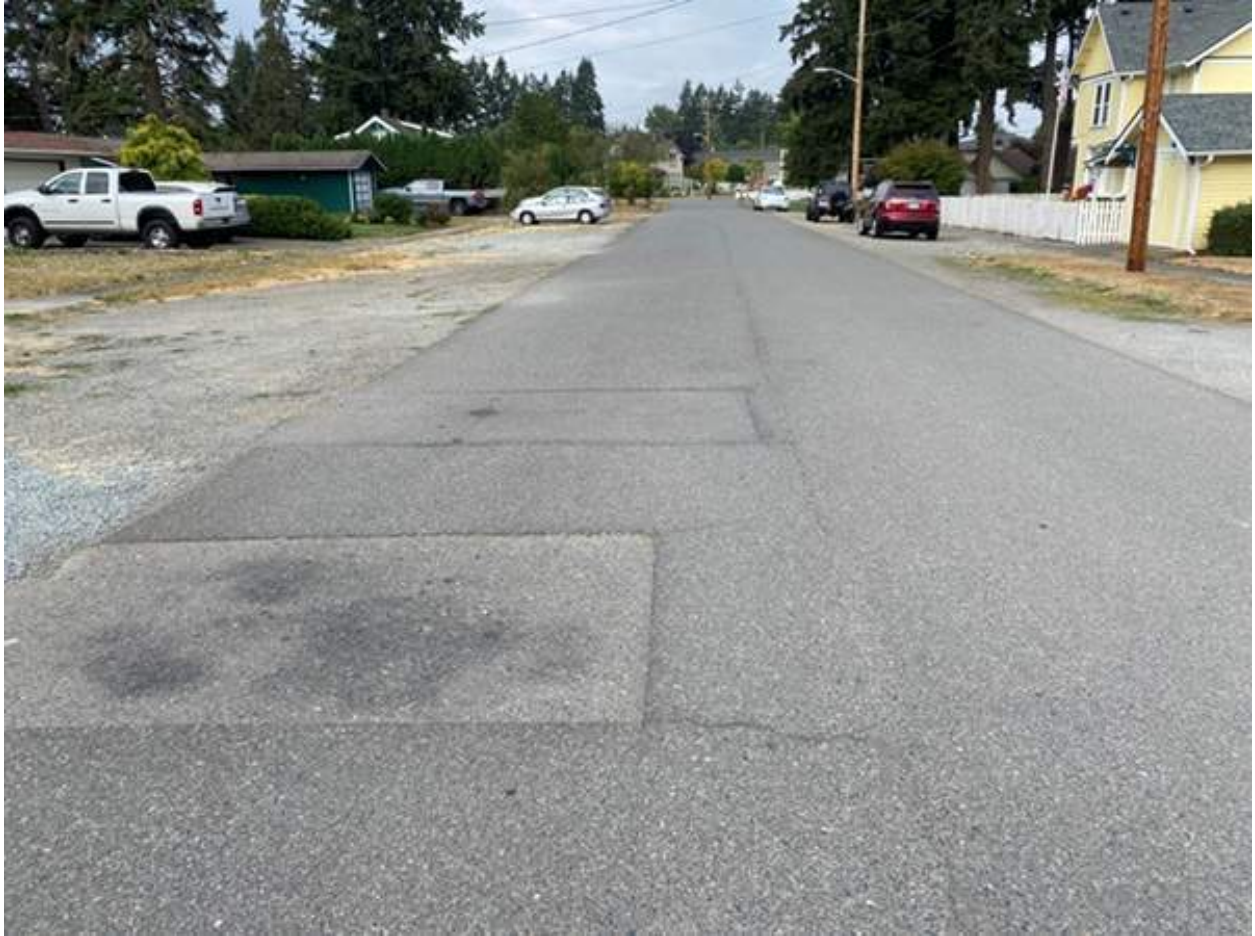
Figure 27. Patching on Bridge Street
