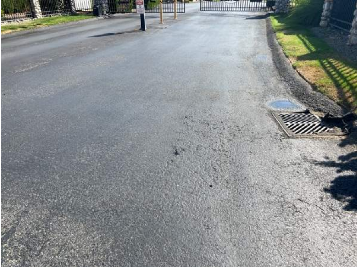
Figure 24. Flushing and Bleeding on Park Place
