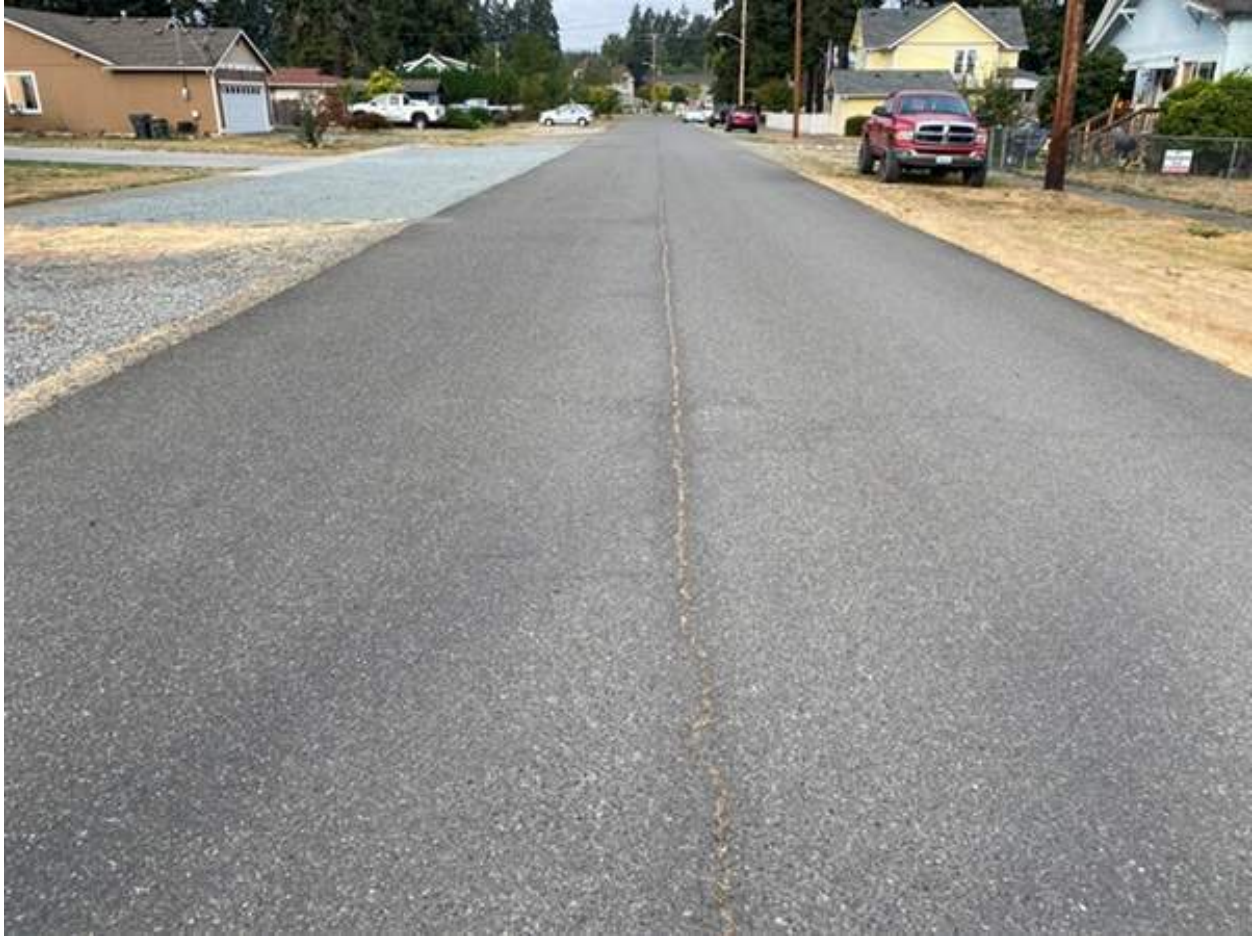
Figure 15. Longitudinal Non-Wheelpath Cracking along Bridge Street
