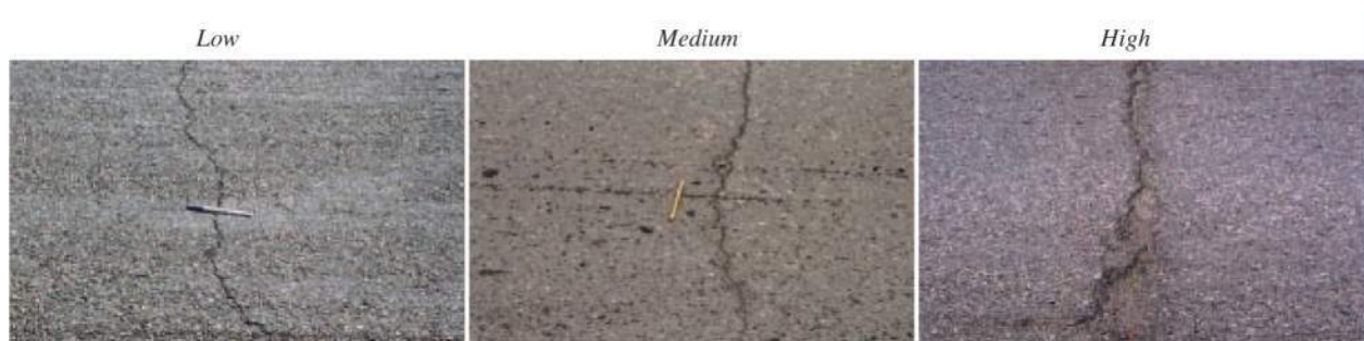
Figure 17. Transverse Cracking Severities
