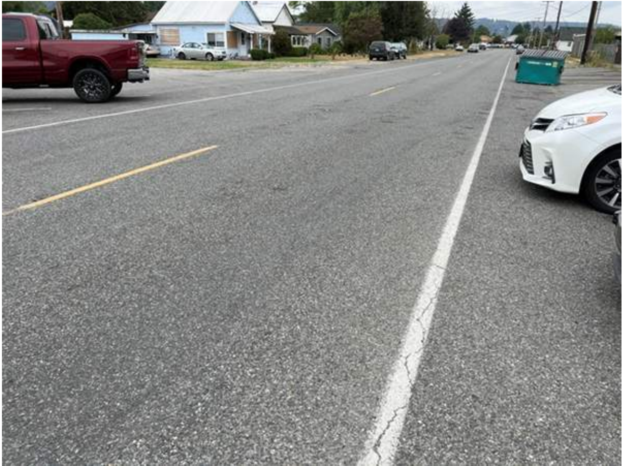
Figure 21. Raveling and Aging along Corrin Avenue
