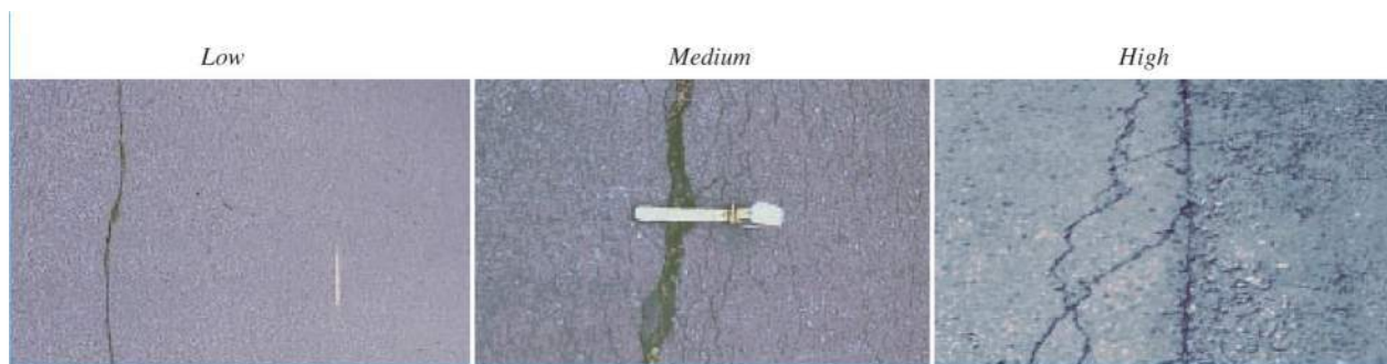
Figure 14. Longitudinal Non-Wheelpath Cracking Severities
